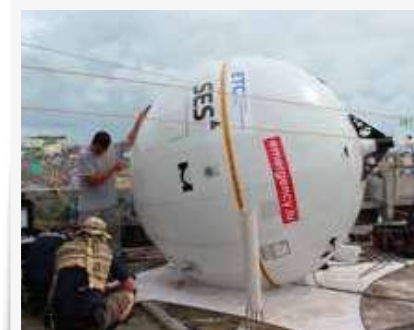
Installation of satellite communications to support the response in the Philippines 2013.
