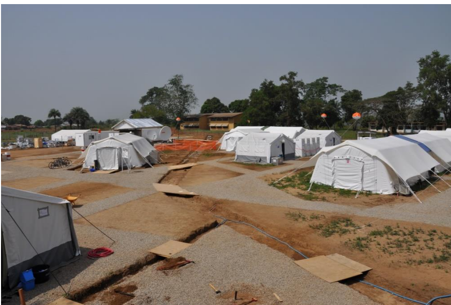
Construction of the IHP Base Camp in Port Loko, Sierra Leone, 2015 (Ebola Outbreak).
